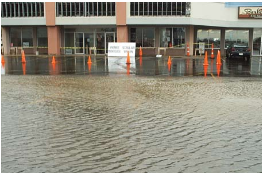
Landmark Plaza experienced severe flooding after summer rain events in 2004 and 2008.
