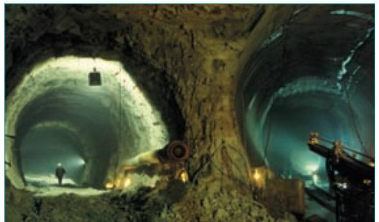
The Deep Tunnel has treated more than 950 gal of CSO.
