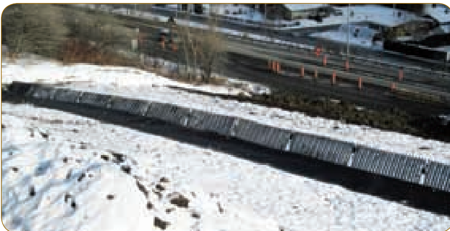
A subdivision at the top of a roadside slope in Quebec generated erosive storm water runoff, requiring the province's Ministry of Transportation to implement a drainage solution.
