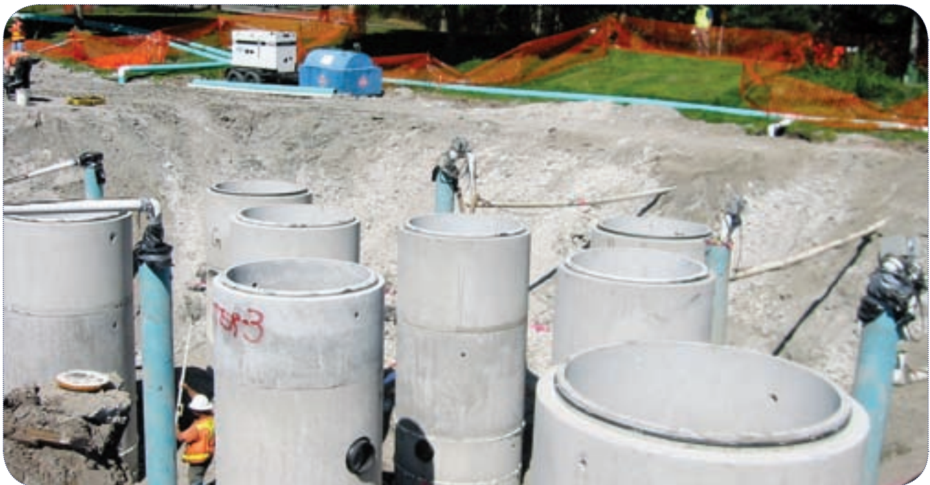
The McRedmond RWQF utilizes a gross particle separator and a storm water filtration system for runoff treatment.
