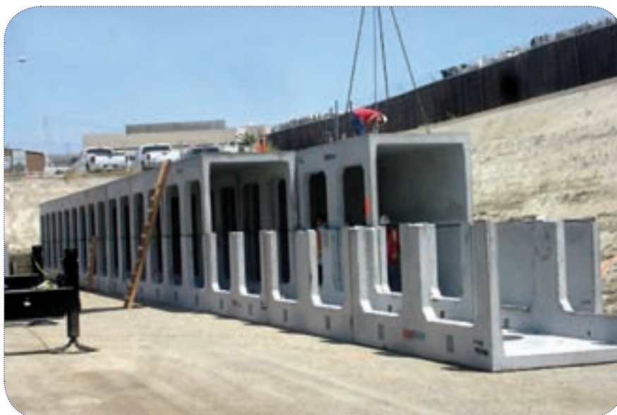
A precast concrete underground retention/detention system helped maximize field area and meet water quality requirements.
