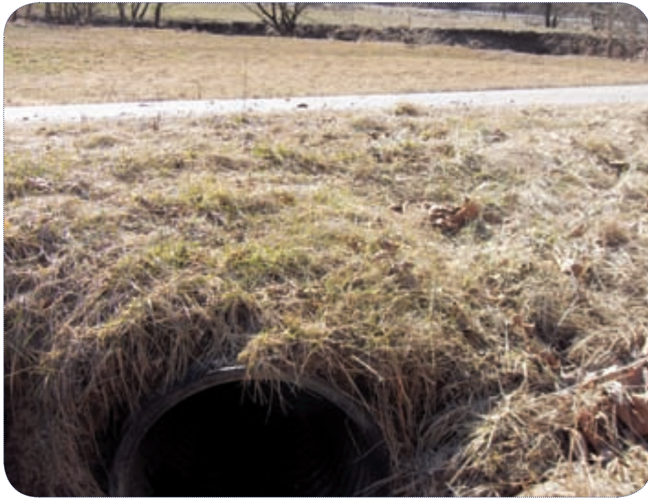
The HDPE pipe runs under Rte. 145 and collects acidic runoff from abandoned strip mines.
