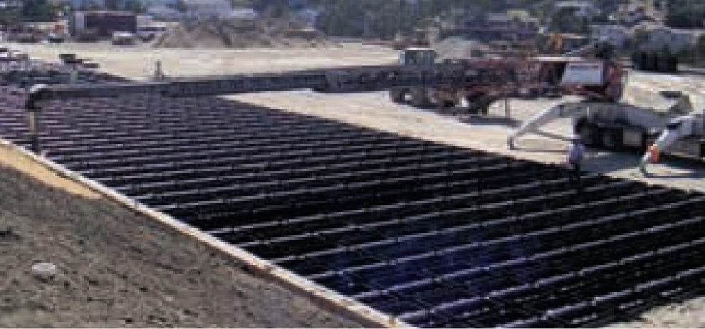
Rainwater and runoff are collected and stored in a 2.2-million-gal subsurface detention basin until needed for irrigation.
