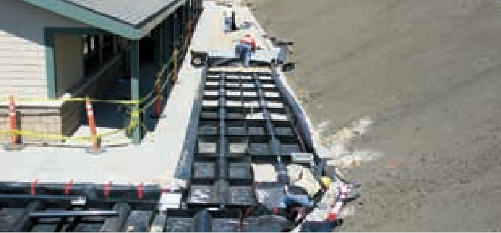
The subsurface irrigation system functions as a collector, water distributor, filtration system and irrigation system.
