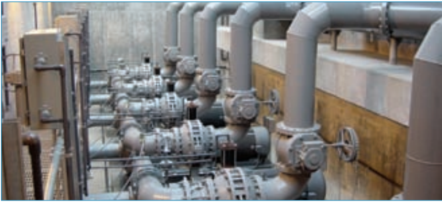
Pumps in the 36-mgd lift station that is the primary feed to the WWTP.
