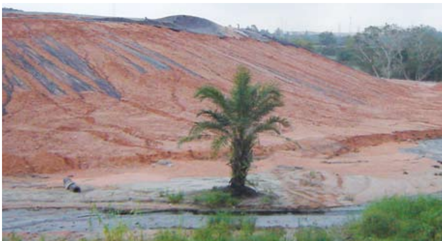
Heavy rain exposed the geomembrane on a Brazilian residue waste slope.
