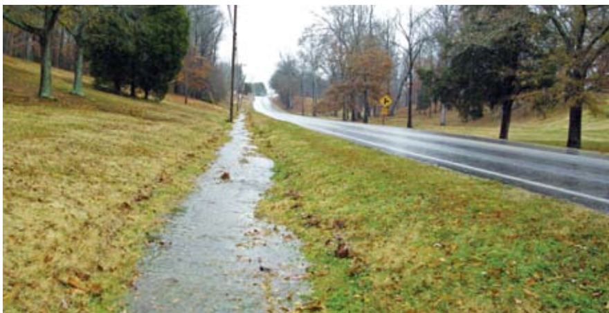
An Alabama roadside storm water ditch before (top) and after (bottom) TRM/geocellular systems.
